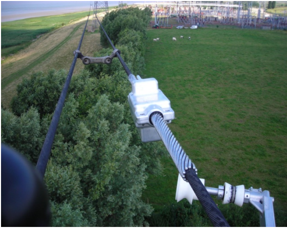
Figure 04: Ampacimon sensor as installed on 400 kV twin conductor line on ELIA's network.
